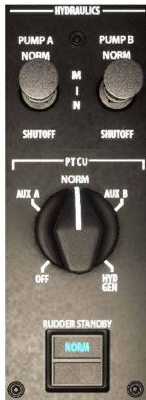
Fig 13-3-1 Hydraulics system controls
